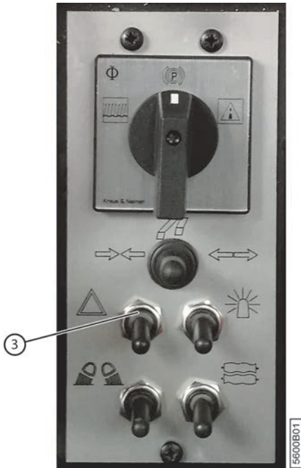
Fig. 63: Switching ON the hazard lights
